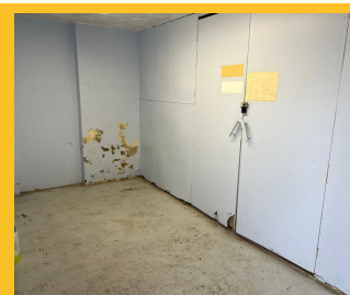
Above: The Swimming Pool changing rooms are currently being refurbished. This 'before' picture illustrates the mess they were in.
